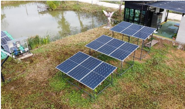
Fig. 2 The PV panels installed at 1 meter, 1.5 meters, and 2 meters
